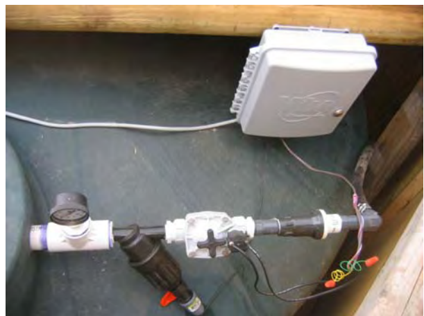
Controls and valves were installed inside of the enclosure.
