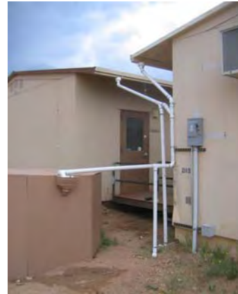
The tank is installed in a plywood enclosure and two roofs are piped with first flush diverters
