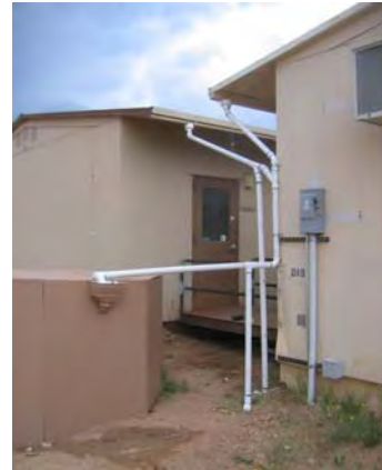
The tank is installed in a plywood enclosure and two roofs are piped with first flush diverters
